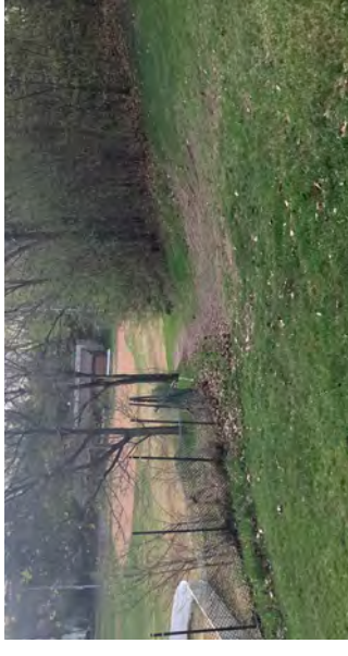
Existing hillside showing erosion on non-accessible route.
