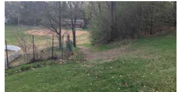
Existing hillside showing erosion on non-accessible route.
