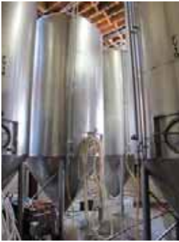
Stainless Steel Tanks for Fermentation
