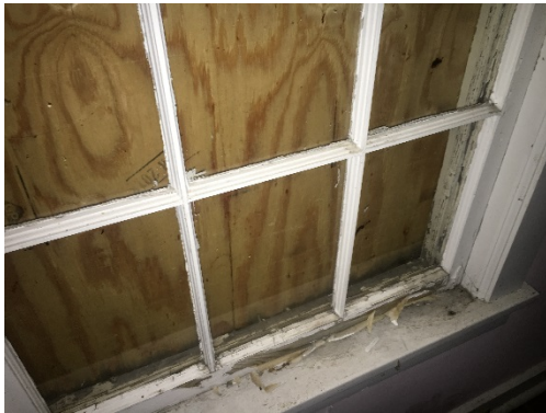
Fig. 1.17 Deteriorating glazing compound at window in upstairs west bedroom
