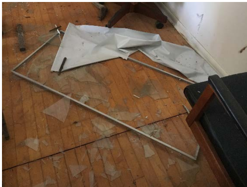
Fig. 1.57 Transition line in hardwood floor in living room at area of second addition
