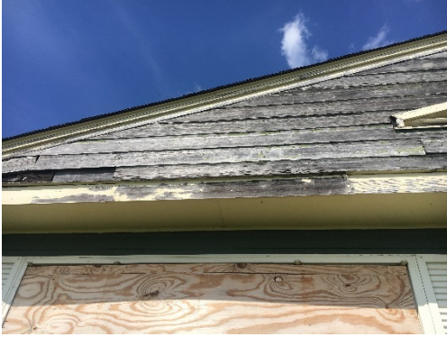
Fig. 1.13 Southern wood clapboard siding with significant peeling paint and weathering
