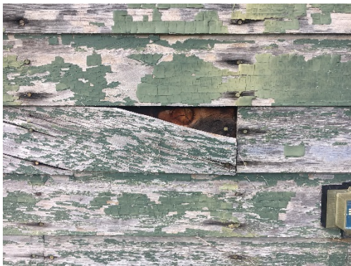
Fig. 1.12 Missing shiplap on east façade
