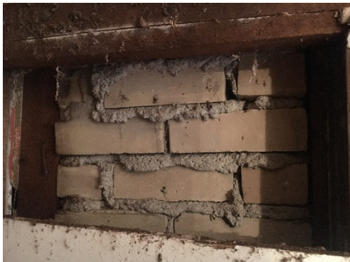
Fig. 1.28 Interior Chaska cream brick chimney at hallway demolition area with unfinished joints
