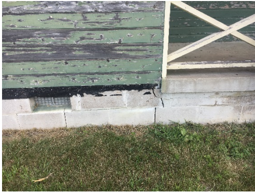
Fig. 1.10 CMU block foundation at porch and south end addition. Note crack at porch.
