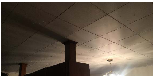
Fig. 1.51 Acoustic ceiling tile in kitchen
