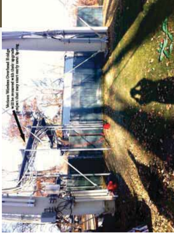
Current Picture of Telecom Site
