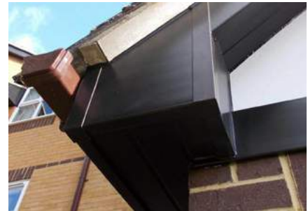
Fig. 3.49 'Porkchop' eave returns are prohibited.
