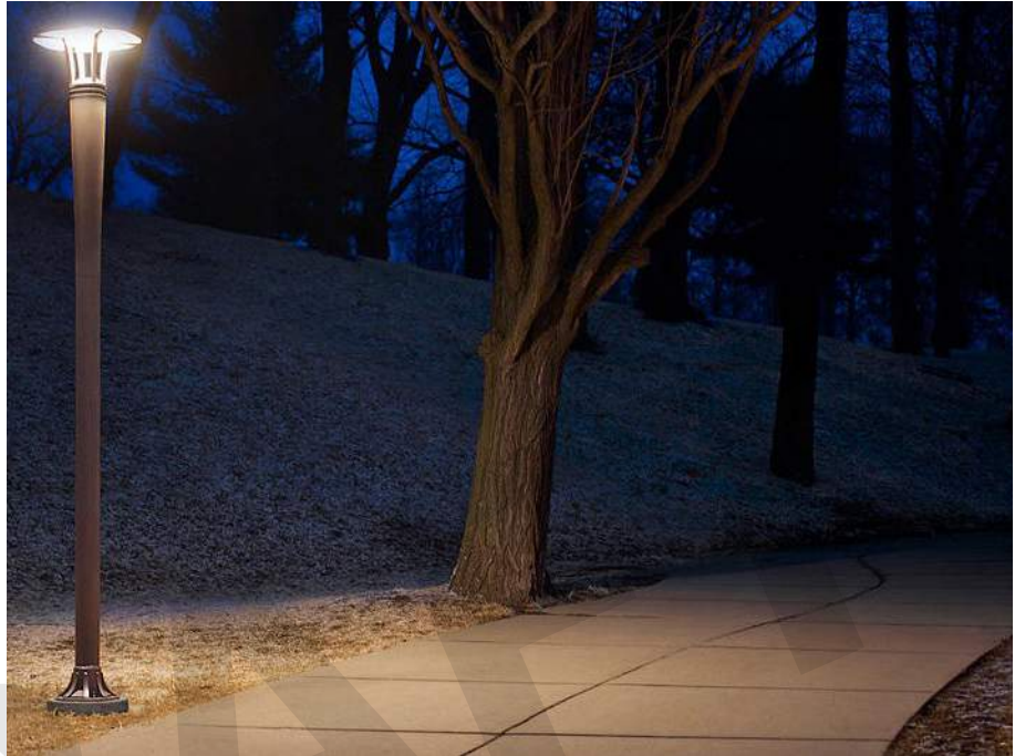
Fig. 2.25 Pedestrian-scale and parking lot site lighting contributes to reducing light pollution by using fixtures with minimal backlight, uplight, and glow.
