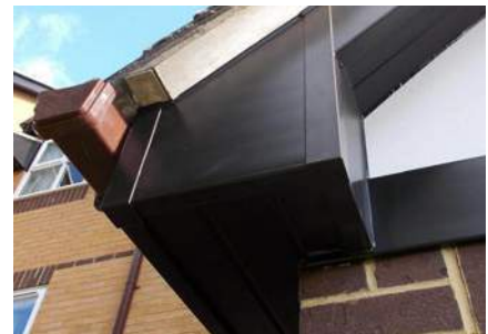
Fig. 3.48 'Porkchop' eave returns are prohibited.
