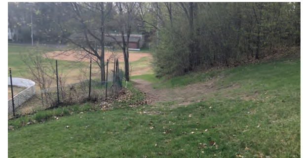
Existing hillside showing erosion on non-accessible route.
