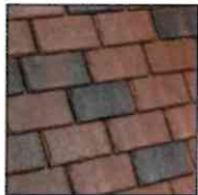
SYNTHETIC SLATE SHINGLE ROOF:
