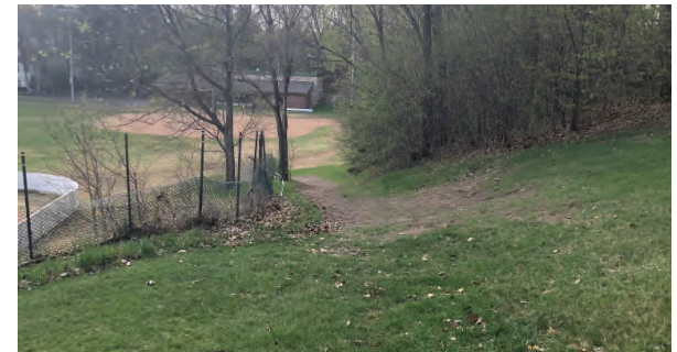
Existing hillside showing erosion on non-accessible route.
