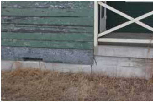
Figure 1.10 CMU block foundation at porch and south end addition. Crack at porch.
