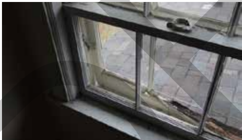
Figure 1.18 Interior view of smaller wood window in upstairs east bedroom. Deteriorating wood at bottom rail
