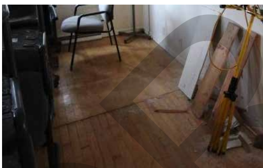
Figure 1.60 Transition line in hardwood floor in living room at area of second addition.
