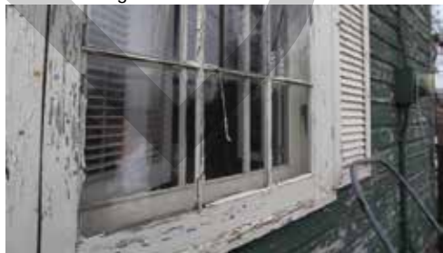
Figure 1.19 Deteriorated glazing compound
