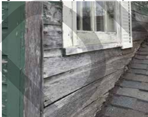
Figure 1.13 Southern wood clapboard siding with significant paint peeling and weathering.
