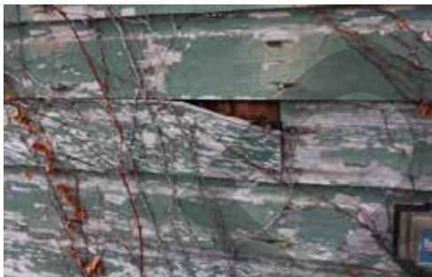
Figure 1.12 Missing shiplap on east façade
