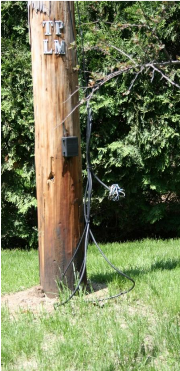
493 Ferndale Road S – Drops not properly attached to the pole
