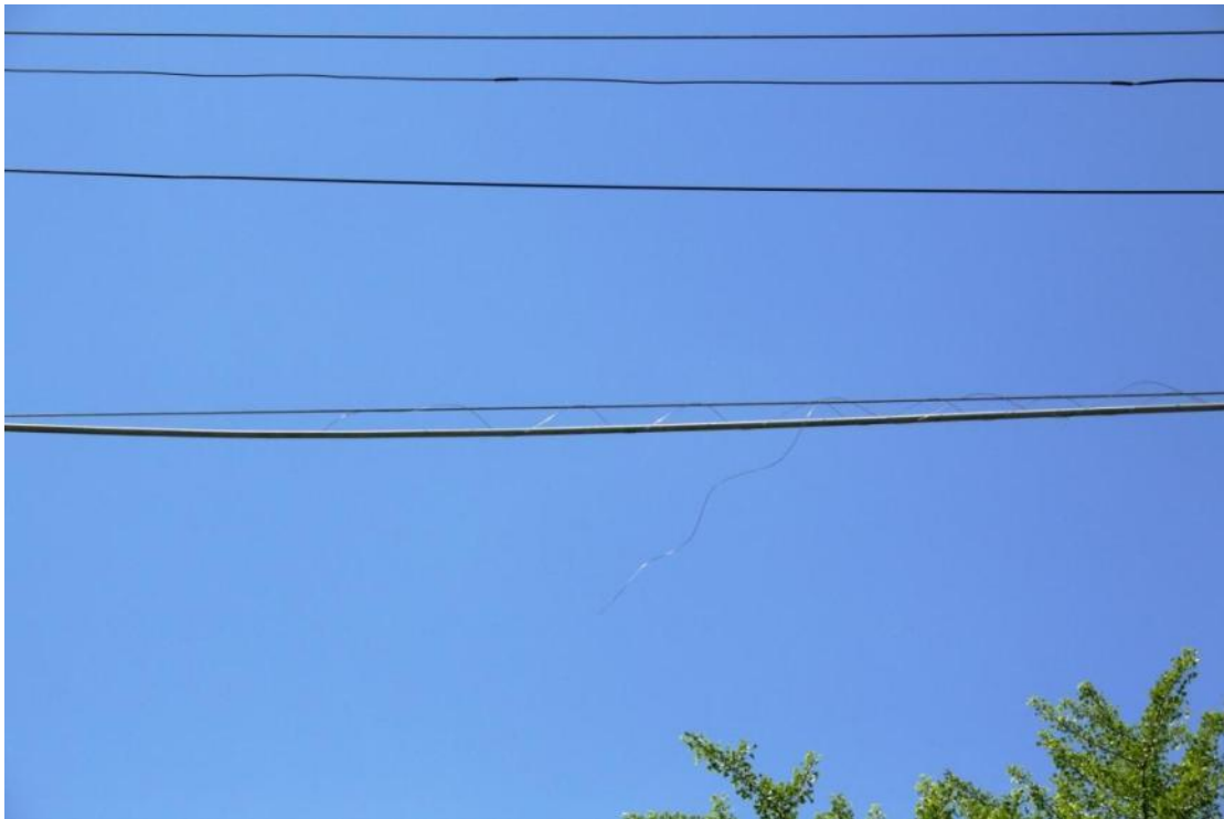
487 Ferndale Road S – Lashing wire is broken and cable is sagging from the messenger
