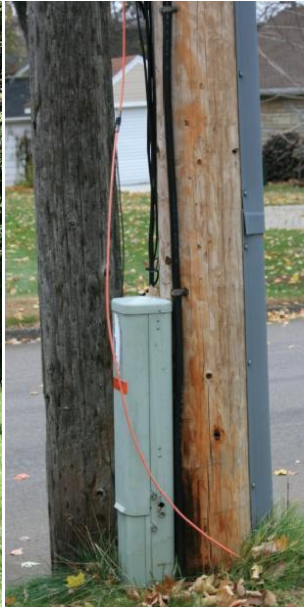
740 Park Street E – Drop not properly attached to the pole
