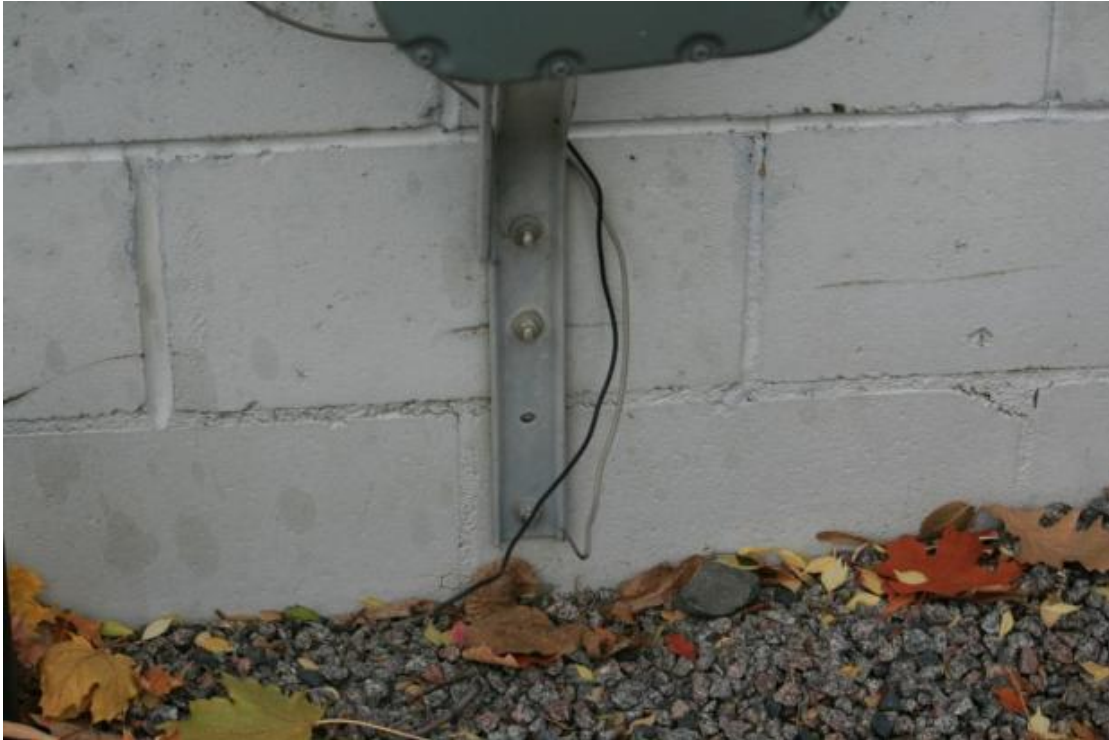
130 Chicago Avenue – No ground or bond (wires are not connected to anything)
