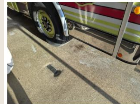
Insufficiently sized floor drain in apparatus bay.
