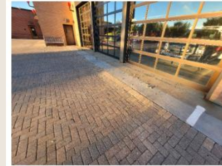
Settled pavers at apparatus bay apron.
