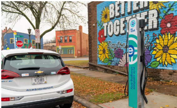
Public EV charging station (Image source: City of Minneapolis)
