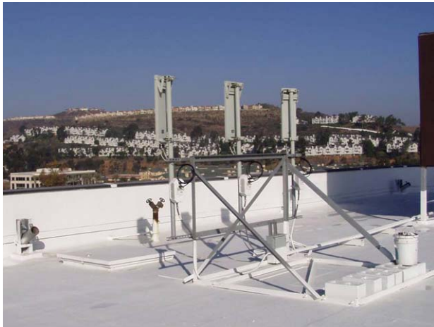
Roof mounted antennas
