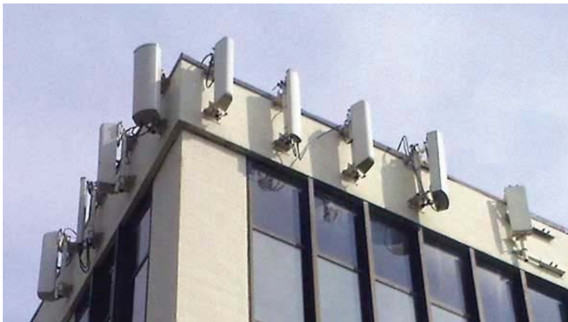
Antennas mounted to the façade of a building
