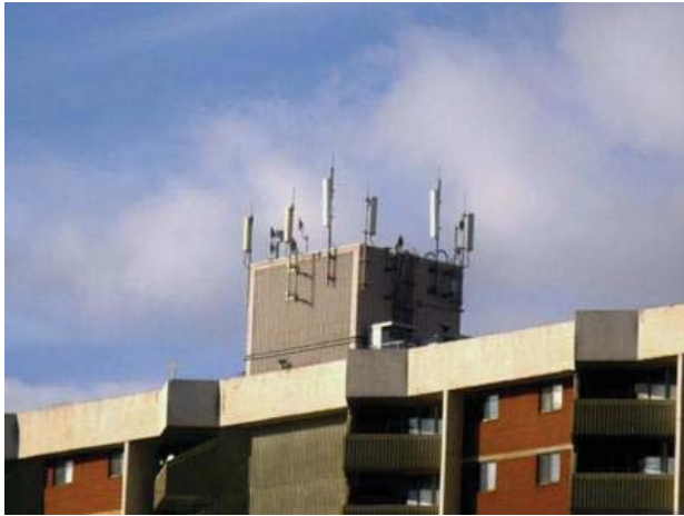
Antennas mounted on top of a mechanical room
