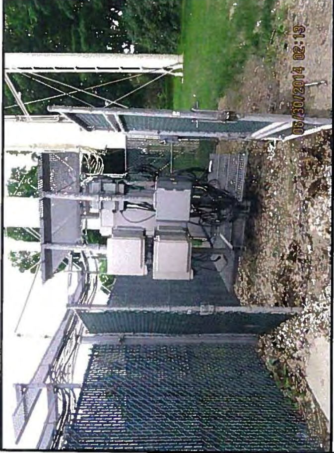
1 EXISTING T-MOBILE EQUIPMENT PLATFORM
